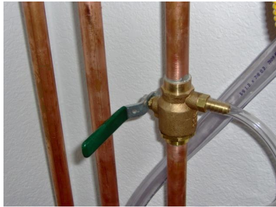
Water valve in "off" position
