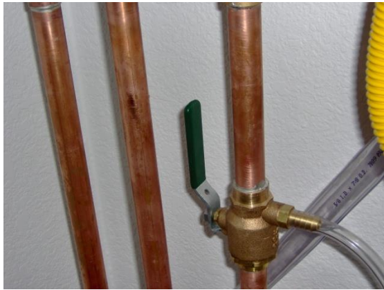
Water valve in "on" position
