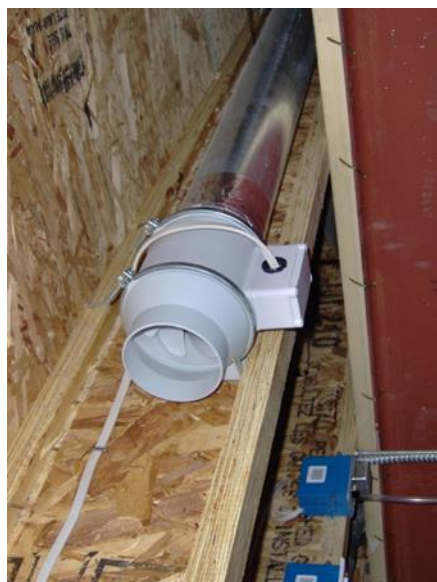
Figure 10 Crawl Space Fan
