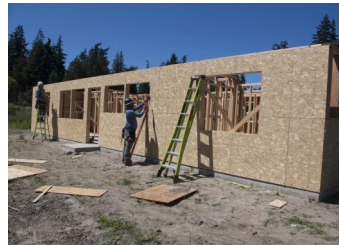
Volunteers work on a home on East Eugene Street in Port Hadlock
