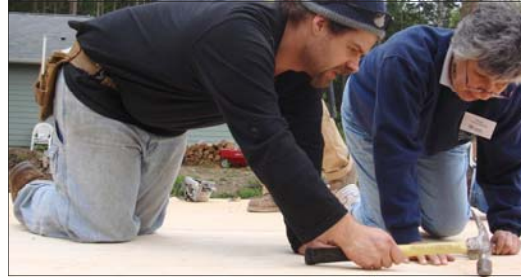
Special events help tell the Habitat story — building houses in partnership with people in need. Here Olympic Community Action trainee James Gray works with volunteer Sheila Khalov on sub flooring for the Leckenby house
