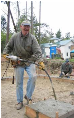
Assistant Site Supervisor Jack Rigger tickles the concrete to remove air bubbles.
